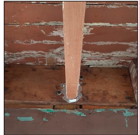
Photo 8: Typical Guard Post Connection
