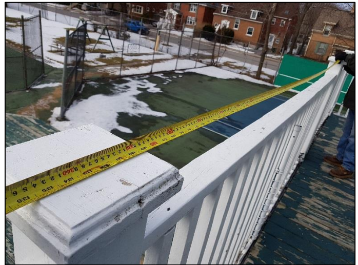
Photo 7: Existing Wood Guards Surrounding Deck
